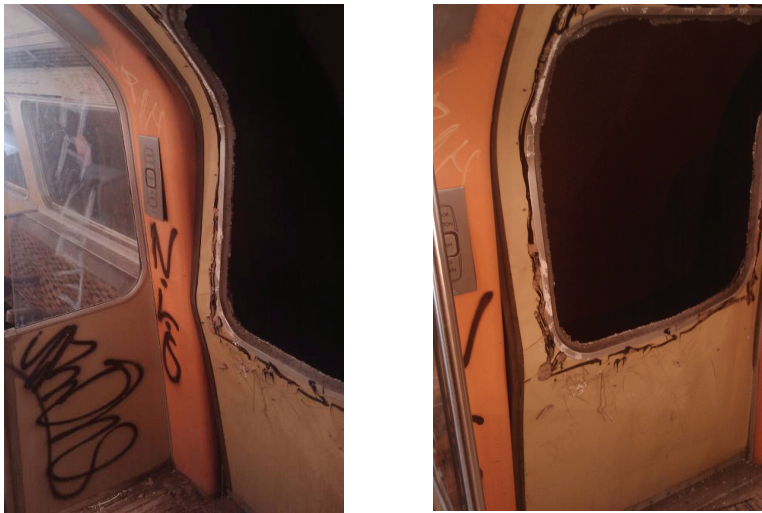
Fig. 4. (a) &(b) Part of a metro vehicle door forced into the compartment due to reflected pressure waves from surrounding tunnel infrastructure.
