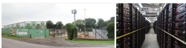
Figure 1: A picture showing the site of the storage (left) and the battery racks (right)
