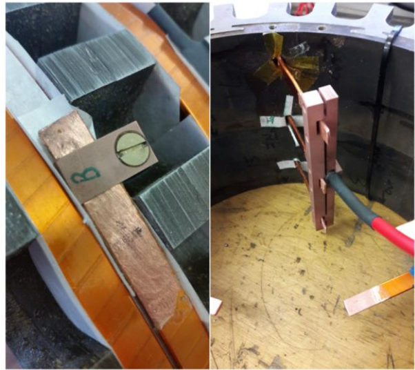
Fig. 10. Copper Clamp for Coil Exit (l) and Busbar Star-point (r) Prior to Covering with Kapton® Insulating Tape
