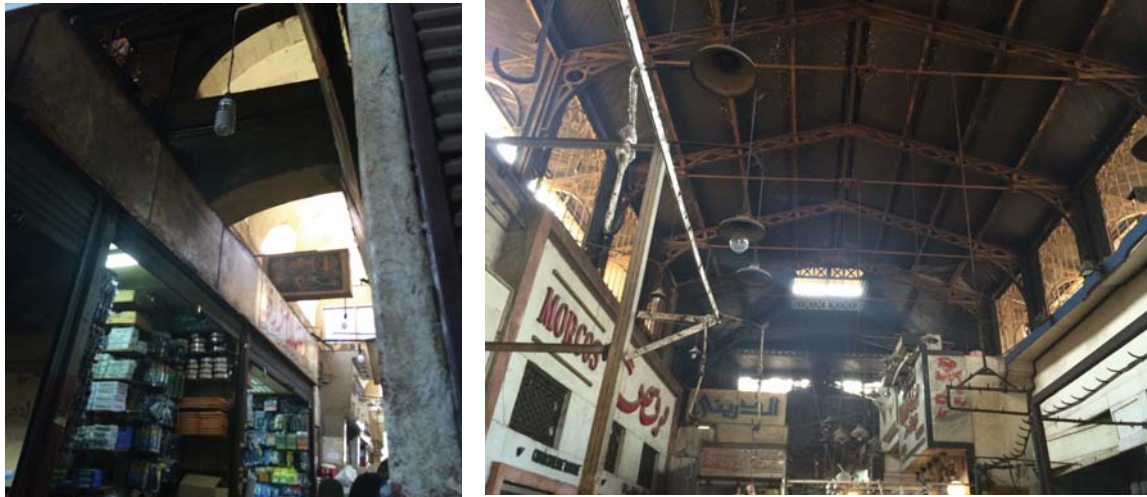
Figure 5. The Clerestory to provide natural daylight and ventilation inside the building: Left, the secondary alleyways; Right, the main Alleyway trusses and side openings (Source: author's collection).
